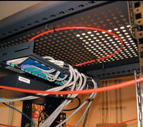
Firetrace does not occupy valuable rack space. This red Firetrace Detection Tubing is run unobtrusively across the top of the rack.
