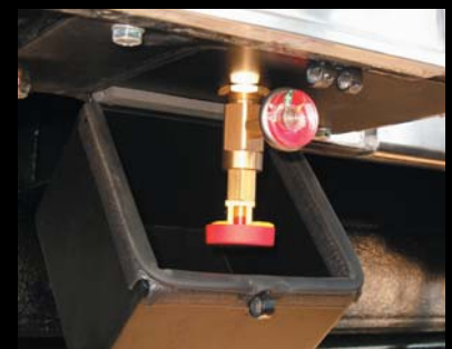
Adjacent to the shredder operation console is this manual release, which enables the operator to operate the system at the first sign of trouble.
