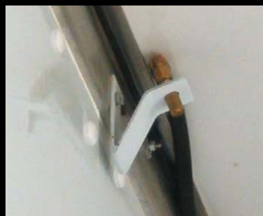
This is one of the nozzles positioned in the collection area, ensuring fast, even delivery of the fire suppressing agent.
